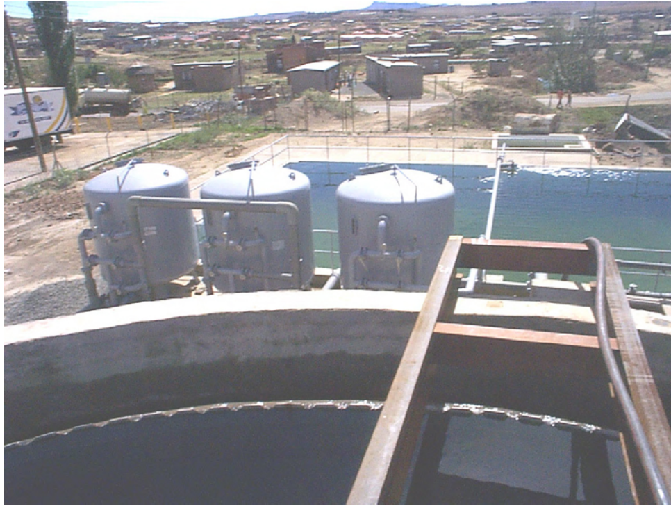
Plate 8: Water recycling plant at a factory in Maseru: significant savings are being made
